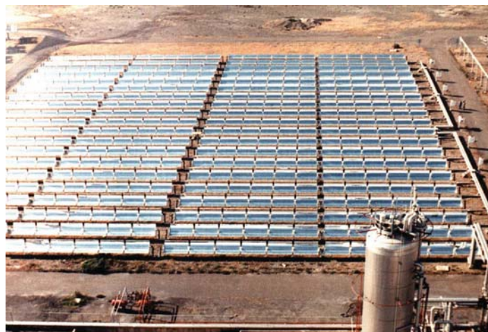
Figure 3: View of solar field of ACUREX facility.
